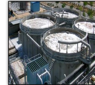
Moving Bed Bio Reactor (MBBR)
