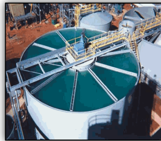
High rate solid contact clarifiers
