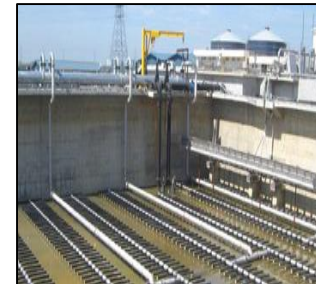
Sequential Batch Reactor (SBR)
