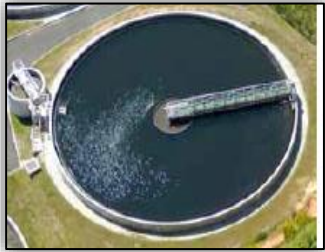
Clarifiers and Clariflocculators
