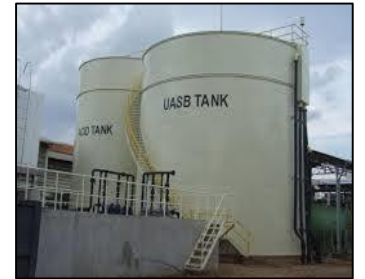
Upflow Anaerobic sludge blanket reactor (UASB)
