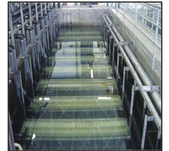
Membrane Bio reactor (MBR)
