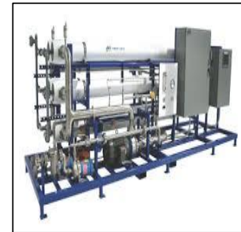
Forward Osmosis (FO) System
