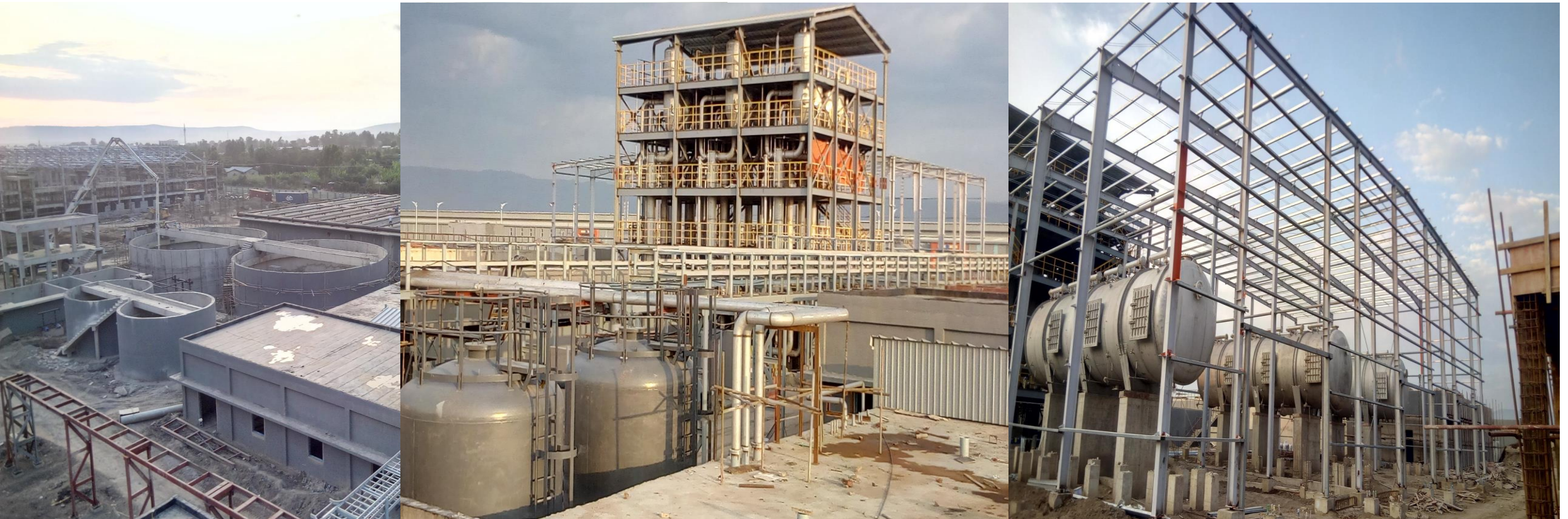
11 MLD Zero Liquid Discharge Plant at Hawassa Industrial Park, Ethiopia
